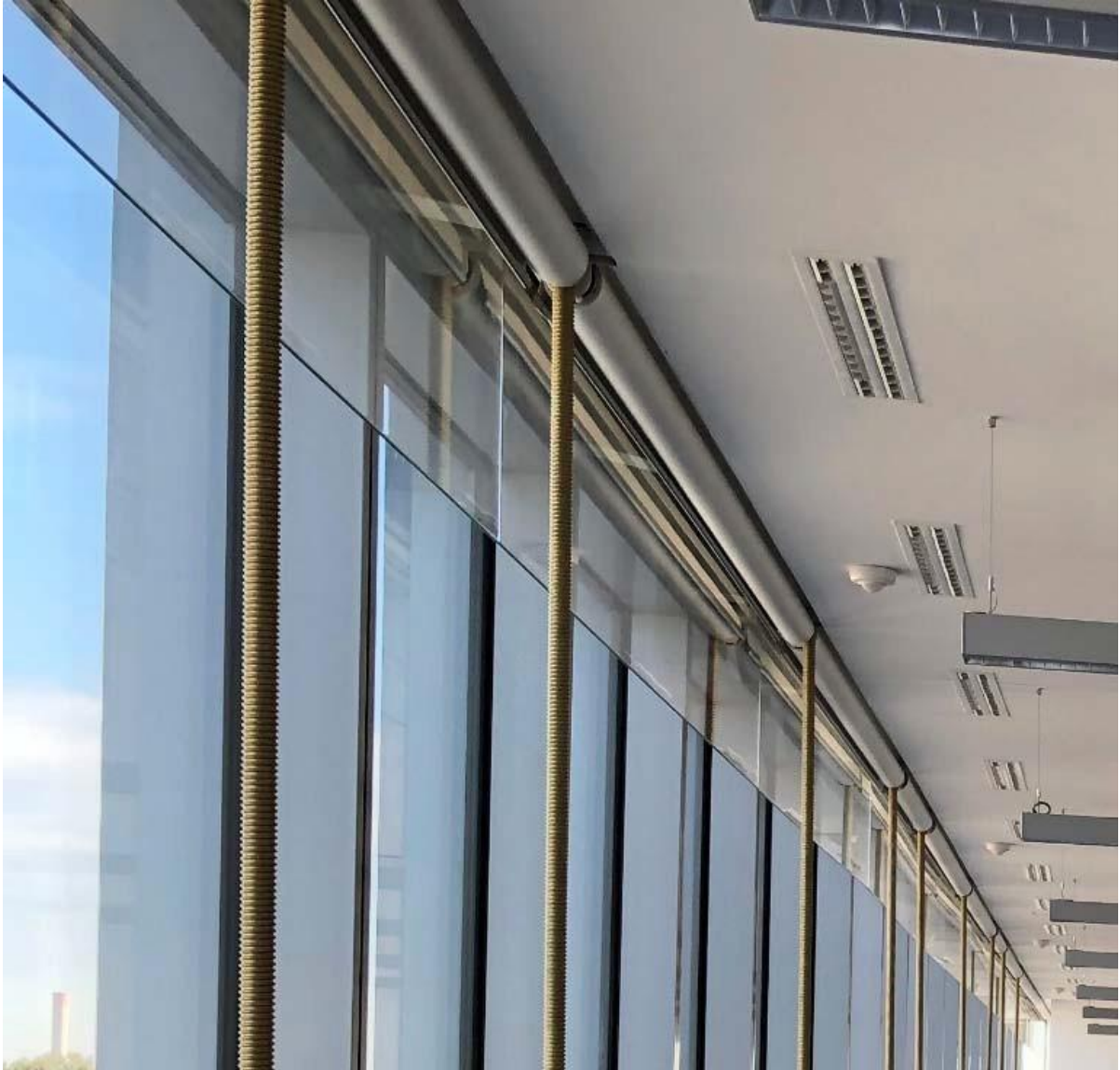
The unique certified glass structure of the façade fire barrier in the “bridge” area with its gold-coloured suspension rods that serve to limit deformities in the ceiling edge.
