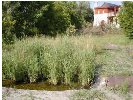
Figure 30: Reedbed sewage treatment in Vácrtót, Hungary
